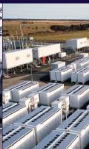
Battery Storage Farms
